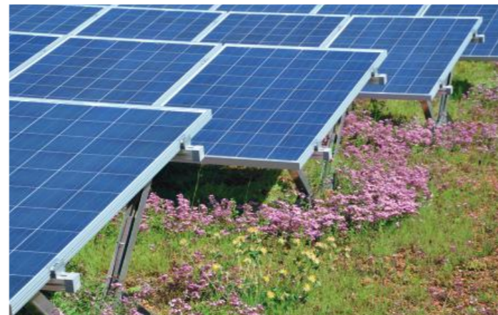
PV panels on green roof mat
